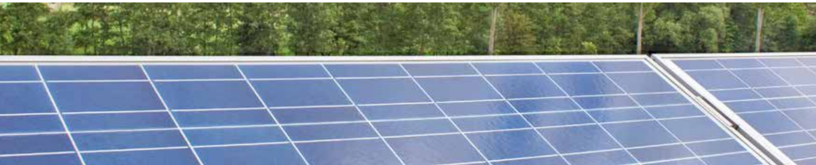
PV Anlage Heinsberg 1,0 Mwp
